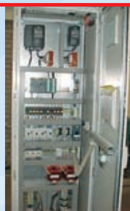
Up to 4 Cleaners on 1 Control System
