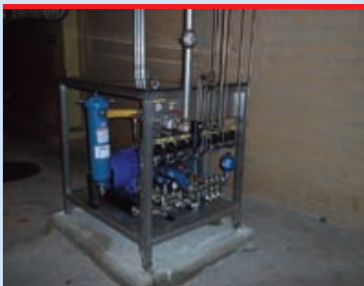
Up to 4 Cleaners on 1 Pumpstation
